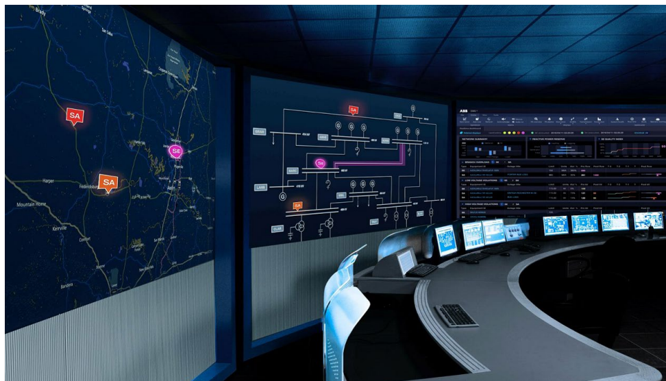
Image from: https://news.cision.com/abb-power-grids/i/control-room,c2661365
